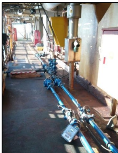
Figure 8 – Scott J17 OOR Pilot hard piping system.
